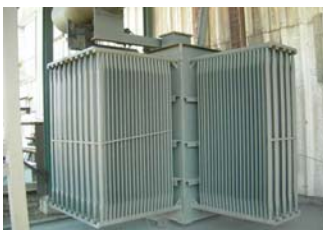
Westinghouse rectifier transformer
