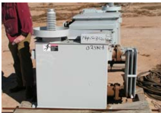
NWL Transformer/Rectifier, 80.2 KVA
