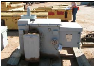
NWL Transformer/Rectifier, 80.2 KVA
