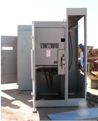
Matra Transformer, 500 KVA
